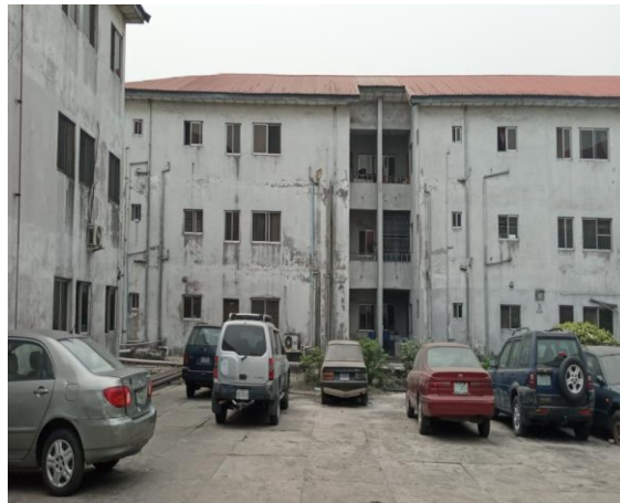
Plate 1: Marine Base Civic Servant Quarters showing the Physical Condition of the Buildings
